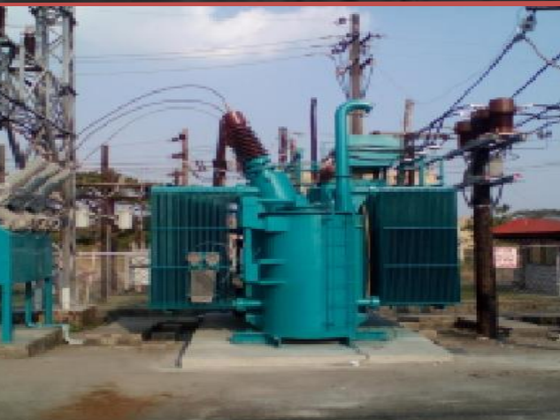
RELOCATION OF 12.5 MVA TRANSFORMER AT DIAMANTE SUBSTATION CLIENT: CLARK ELECTRIC DISTRIBUTION CORPORATION (CEDC) LOCATION: CLARK, PAMPANGA SCOPE OF WORKS: ELECTRICAL WORKS
