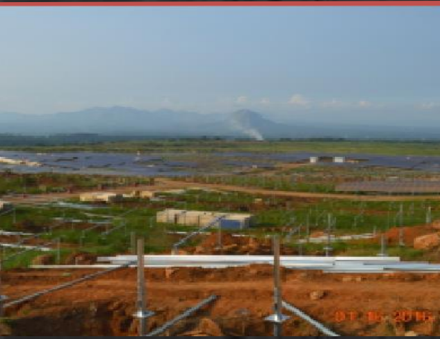
14.5 MVA SUBSTATION HERMOSA SOLAR POWER PLANT PROJECT CLIENT: GREEN POWER LOCATION: HERMOSA, BATAAN SCOPE OF WORKS: CIVIL AND ELECTRICAL WORKS
