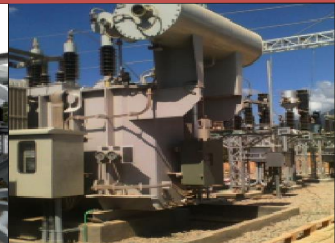
18MVA SUBSTATION AND SWITCHING STATION MARIVELES SOLAR FARM PROJECT CLIENT: MSERV (MERALCO ENERGY INC.) LOCATION: MARIVELES, BATAAN SCOPE OF WORKS: CIVIL AND ELECTRICAL WORKS
