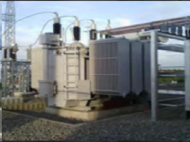
25MVA SUBSTATION AND SWITCHING STATION SILAY SOLAR FARM PROJECT
