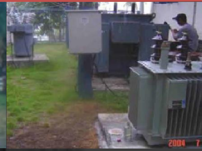
ZUMARRAGA ISLAND ELECTRIFICATION PROJECT POWER GENERATION AND TRANSMISSION (ISLAND GRID) 15KMS
