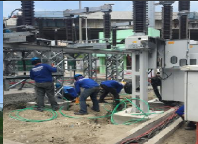
EMERGENCY WORKS OF 115KV IMELDA SUBSTATION INCLUDING THE 1x50MVAR CAPACITOR BANK NO. 2 CLIENT: NATIONAL GRID CORPORATION OF THE PHILIPPINES (NGCP) LOCATION: DOÑA IMELDA SUBSTATION SCOPE OF WORKS: CIVIL AND ELECTRICAL WORKS
