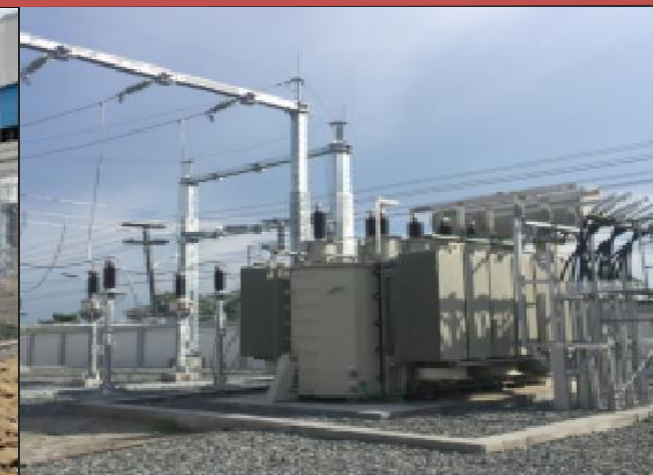
DESIGN AND CONSTRUCTION OF 2X50MVA, 69KV/13.8KV ROXAS SUBSTATION CLIENT: CLARK ELECTRIC DISTRIBUTION CORPORATION / MERALCO ENERGY CORPORATION (MSERV) LOCATION: ANGELES CITY, PAMPANGA SCOPE OF WORKS: GENERAL CONSTRUCTION
