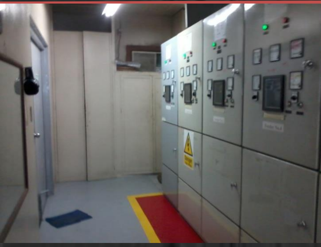
UPGRADING OF LVSG AT AMANPULO ISLAND
