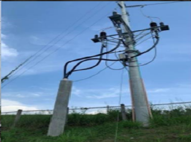
69KV LINES FROM ROXAS SUBSTATION TO IE-5 SUBSTATION PHASE 1 CLIENT: CLARK ELECTRIC DISTRIBUTION CORPORATION (CEDC) LOCATION: CLARK FREEPORT ZONE, PAMPANGA SCOPE OF WORKS: CIVIL AND ELECTRICAL WORKS
