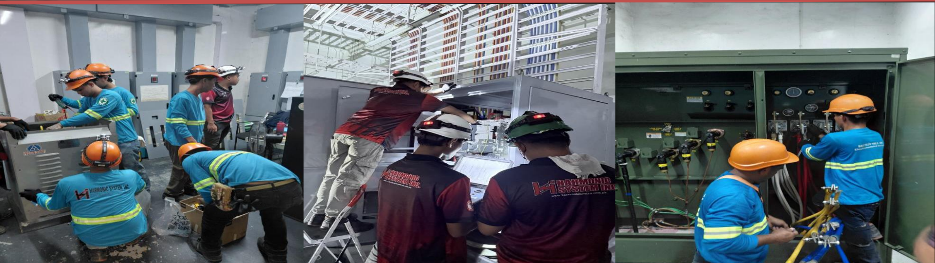
PREVENTIVE MAINTENANCE @ S&R CABANATUAN AND S&R SUCAT
