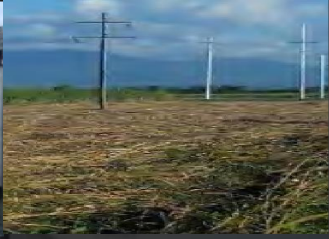
69KV TRANSMISSION LINES FOR SILAY SOLAR FARM PROJECT
