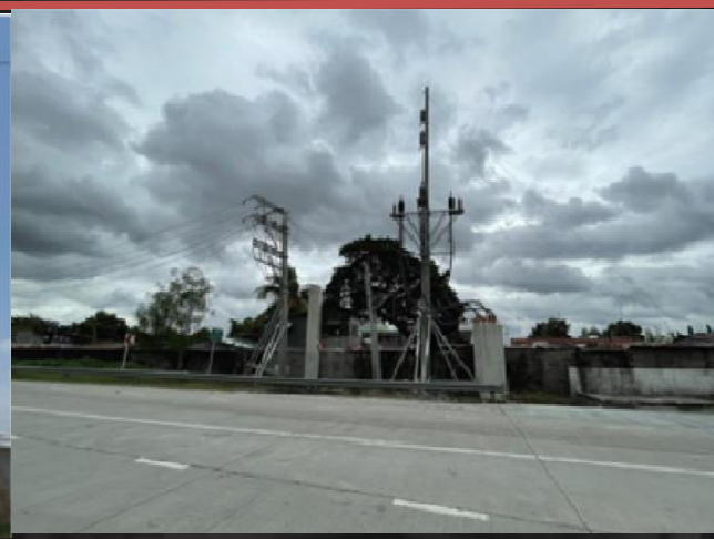
CONSTRUCTION OF 69KV / 13.8KV UNDERGROUND NEAR SM CITY CLARK CLIENT: CLARK ELECTRIC DISTRIBUTION CORPORATION (CEDC) LOCATION: MABALACAT-ANGELES ROAD, PAMPANGA SCOPE OF WORKS: CIVIL AND ELECTRICAL WORKS
