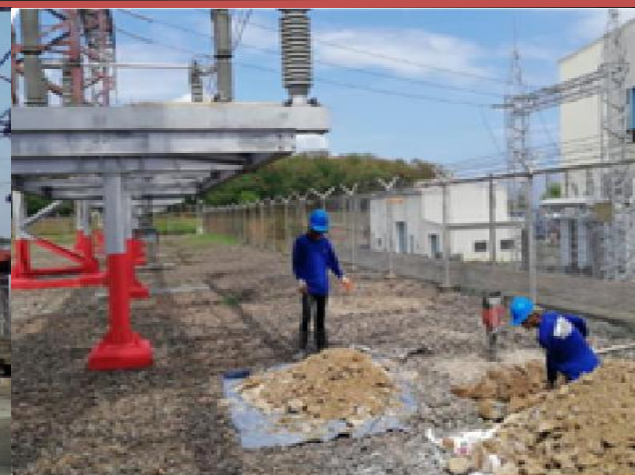
CONSTRUCTION OF METERING FACILITIES OF NGCP @LIMAY BCCP 230KV SUBSTATION CLIENT: NATIONAL GRID CORPORATION OF THE PHILIPPINES (NGCP) LOCATION: LIMAY, BATAAN SCOPE OF WORKS: CIVIL AND ELECTRICAL WORKS
