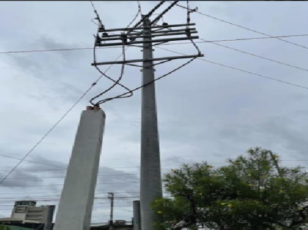
CONSTRUCTION OF 13.8KV UNDERGROUND POWER CABLE ALONG M.A. ROXAS HIGHWAY CLIENT: CLARK ELECTRIC DISTRIBUTION CORPORATION (CEDC) LOCATION: ANGELES CITY, PAMPANGA SCOPE OF WORKS: CIVIL AND ELECTRICAL WORKS
