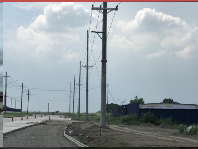
CONSTRUCTION OF 13.8KV LINE GOING TO GARDENIA CLIENT: CLARK ELECTRIC DISTRIBUTION CORPORATION (CEDC) LOCATION: ANGELES, PAMPANGA SCOPE OF WORKS: ELECTRICAL WORKS
