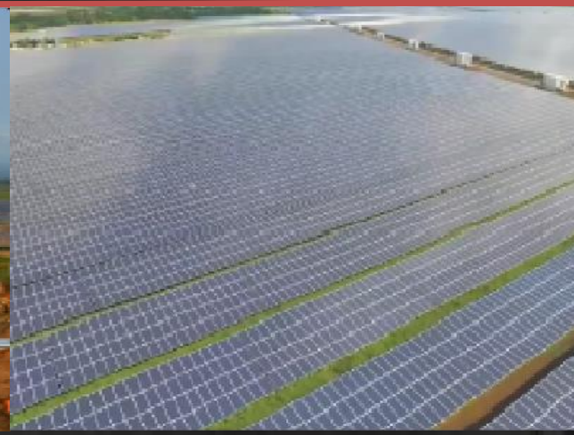
132.5 MW HELIOS POLLO SOLAR POWER PROJECT CLIENT: BOUYGUES / PAMATEC LOCATION: BRGY. TINAMPAAN, CADIZ CITY, NEGROS OCCIDENTAL SCOPE OF WORKS: CIVIL AND ELECTRICAL WORKS
