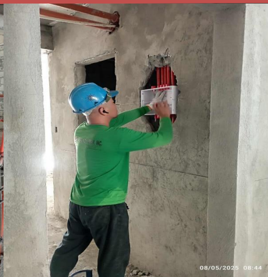
PANELBOARD & BOX SETTINGS @ BLDG. E & F - GF
