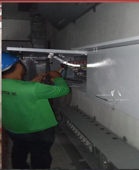
BUSDUCT PLUG-INS TO BUSBAR GUTTER CABLING AND TERMINATION @ GF – 8F EE ROOMS
