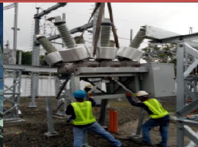
50MVA 69KV/13.8KV SUBSTATION AT KALAW CLIENT: CLARK ELECTRIC DISTRIBUTION CORPORATION / MERALCO ENERGY CORPORATION (MSERV) LOCATION: KALAW SUBSTATION CLARK ANGELES, PAMPANGA SCOPE OF WORKS: GENERAL CONSTRUCTION
